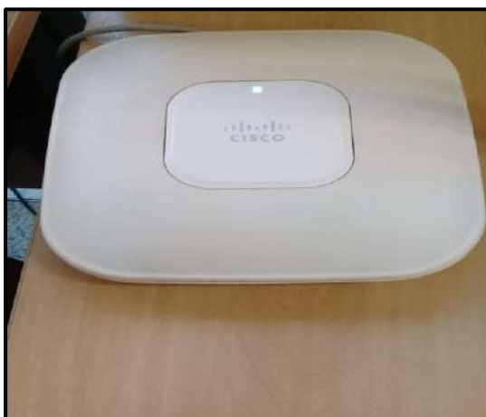
Access point Cisco
